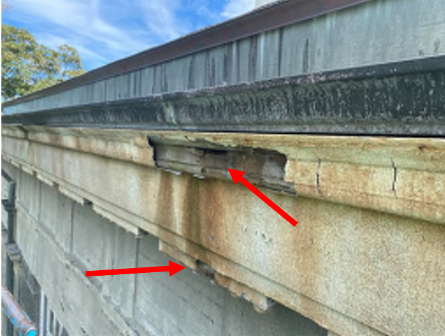
Image 213: Close-up of a missing section of wood trim on top of a pilaster.
