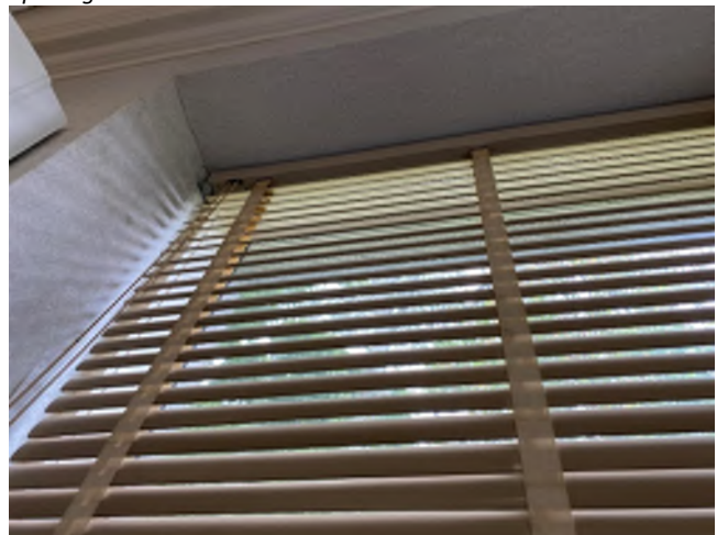
Image 76: The windows within this space utilize blinds with larger slats compared to other spaces. These blinds were difficult to operate.
