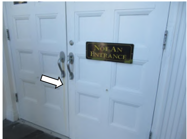
Image 110: The arrow staining emanating from the exterior door hardware.
