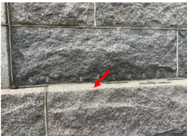
Image 158: Deteriorated and detached mortar on top of the granite foundation.
