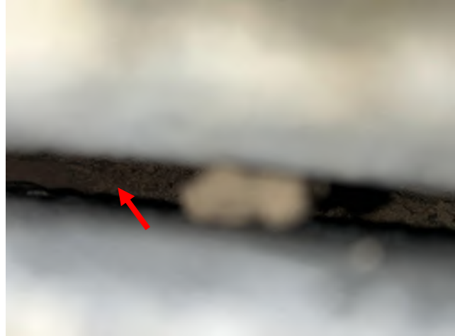
Image 252: Closer view of the previous image shows bedding mortar that appeared to be deteriorated.
