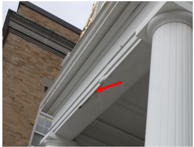
Image 222: Peeling paint on the underside of the façade beam.
