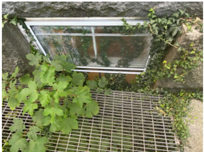
Image 8: Vegetation growth basement window. At this window location, vegetation growth was observed behind the storm window.
