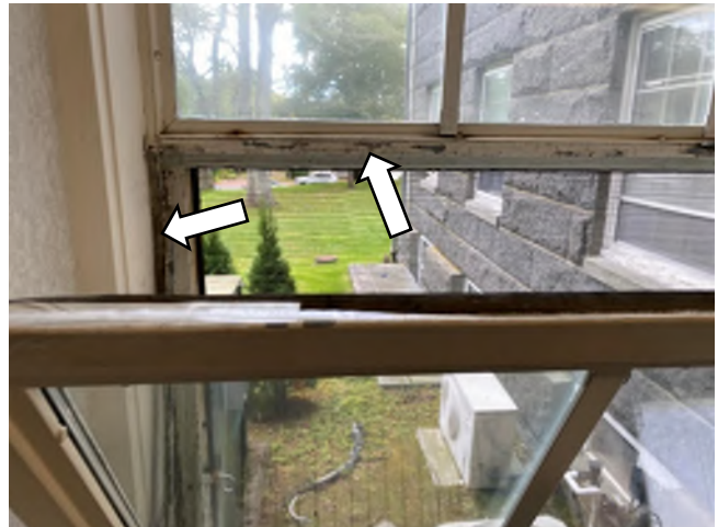
Image 32: The arrow indicates paint defects on the steel window frames common where the hopper sash unit meets the fixed frame.
