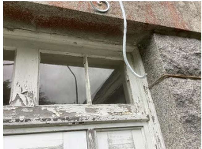
Image 102: The transom utilizes glazing putty to seal the glass and is generally poor condition.
