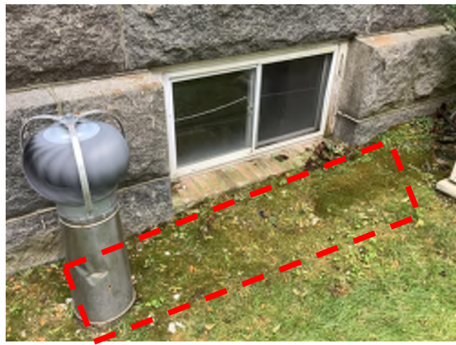
Image 169: Mortar debris had fallen to the ground.
