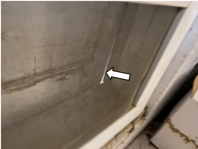
Image 127: The arrow indicates daylight visible between the frame and door when closed.
