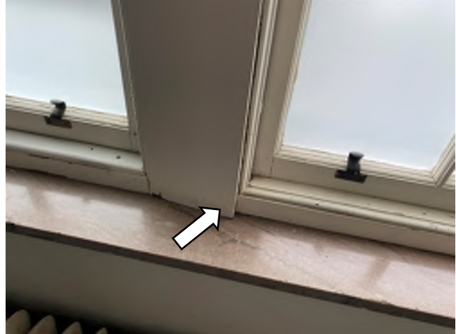
Image 86: The arrow indicates wood trim at the vertical mullion that is warped and displaced.
