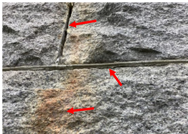
Image 159: Missing/deteriorated mortar joints. Rust staining observed on the granite masonry.
