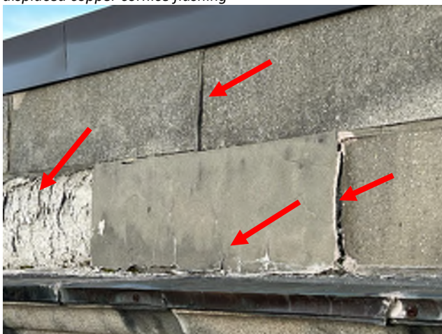
Image 190: Spalled, cracked and delaminated precast components with deteriorated mortar joints on the parapet.
