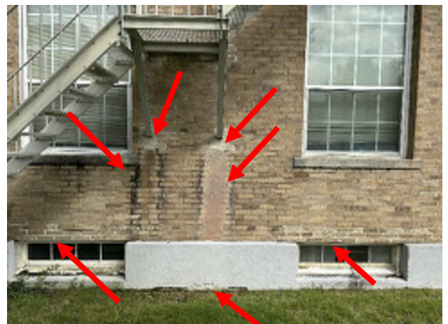
Image 173: Arrows point to black staining, replaced brick masonry units, dissimilar repair mortar and delaminated coating at the base of the wall at grade.
