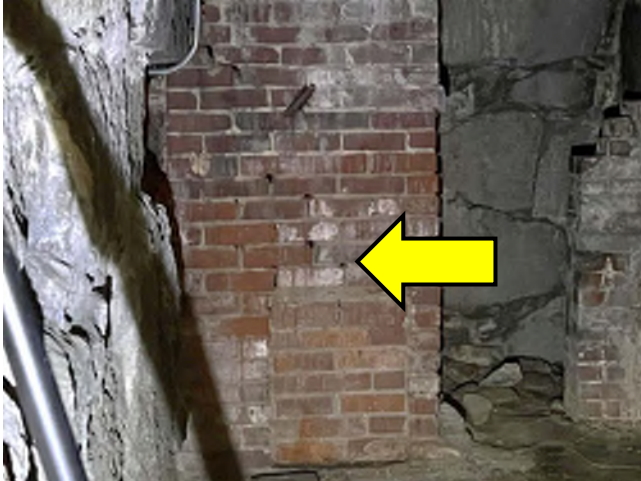
Image 237: View of a step crack and deteriorated masonry in the west masonry wall below the exterior granite steps.
