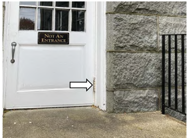
Image 106: The arrow indicates a rusted hinge.
