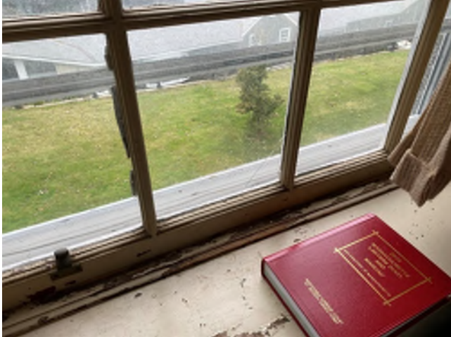
Image 89: Deterioration of interior painted surfaces was noted at multiple openings within this space.
