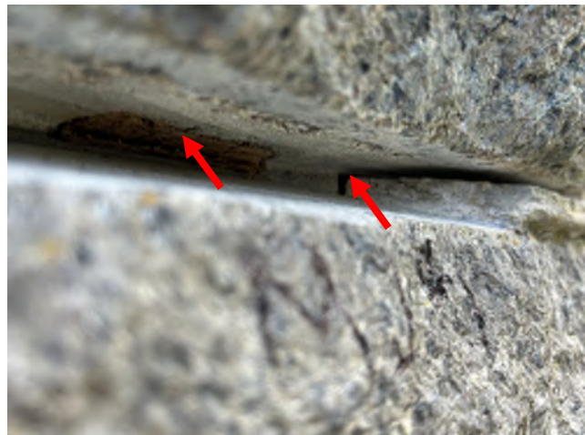
Image 242: Angled view of the previous image shows a clean break between the pointing and bedding mortar, and a metal shim in the bedding mortar at the back of the cut.
