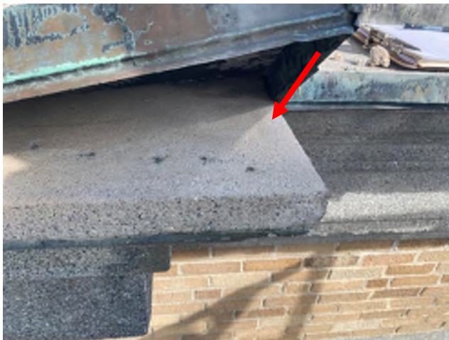
Image 188: Exposed precast cornice section due to loose / displaced copper cornice flashing
