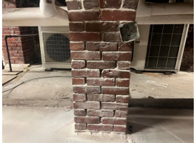
Image 226: Typical view of the deteriorated mortar joints at the base of the masonry piers in the basement of the 1831-1832 building.
