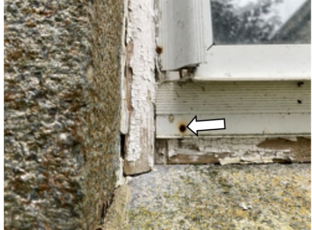
Image 6: Detail view of typical condition of exterior wood trim and sill. The arrow indicates a rusted fastener that secures the storm window to the wood sill.
