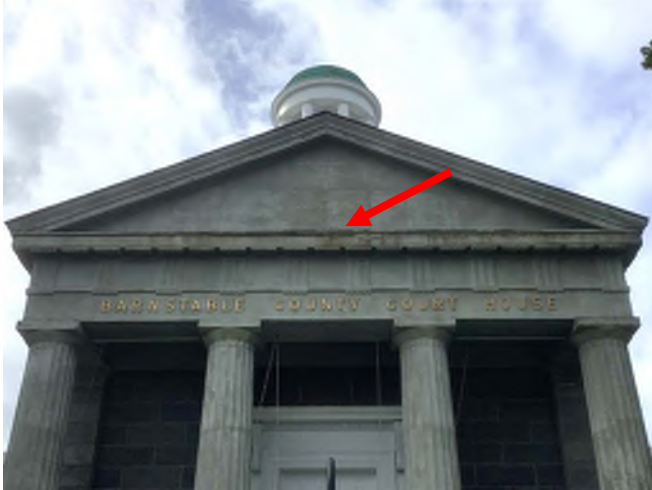
Image 215: View shows deteriorated sand-textured painted surfaces on the pediment elements at the original building's front entrance.
