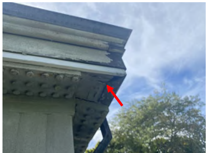
Image 212: View of deteriorated and loose soffit board below the cornice.
