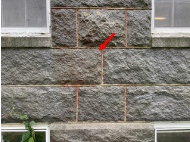
Image 153: View of red algae staining on the rock-faced granite.
