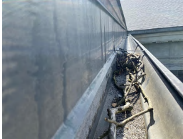
Image 214: View of debris in a copper gutter.
