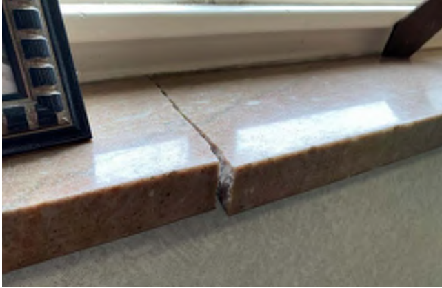
Image 73: An example of a cracked marble stool.
