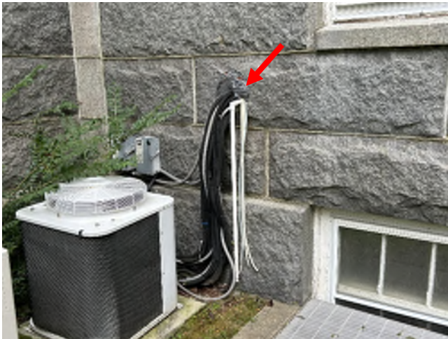
Image 155: Deteriorated spray foam applied to seal numerous conduits that penetrate the granite wall on the east elevation.
