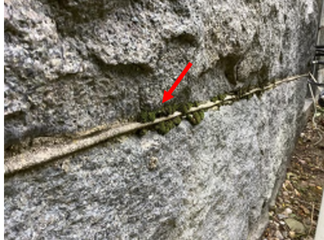
Image 167: Vegetative growth on the granite foundation wall.
