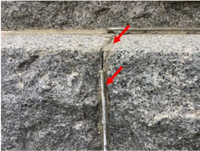
Image 160: Deteriorated and detached mortar, as well as open joints, on top of the granite foundation.
