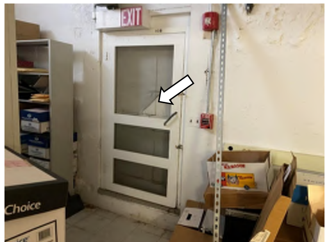
Image 124: Interior view of Door 7 and interior screen door. The arrow indicates damage to the screen.
