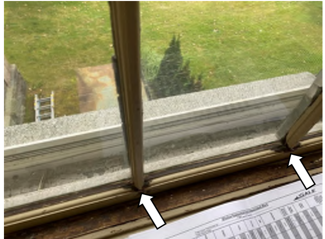
Image 12: At this window location, deterioration was observed where the muntins meet the sash bottom rail (arrows).
