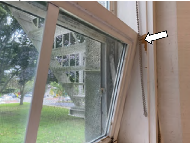
Image 31: The arrow indicates a location where the operable hopper unit sash is rubbing against the wood framing and is eroding the paint layer.
