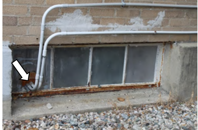
Image 38: Exterior view of the steel basement window. Rust is visible throughout the frame, and the glazing putty is deteriorated. The arrow indicates two (2) conduits installed through a broken pane of glass.
