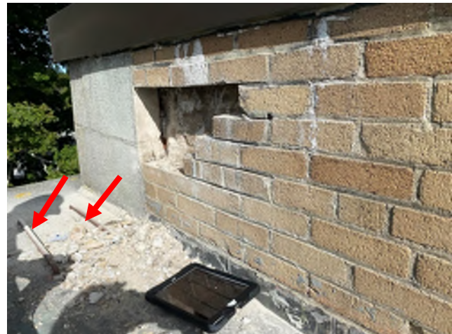
Image 185: Iron anchors (arrows) on the cornice at the left side of the image.
