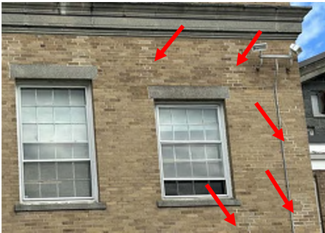
Image 176: Closer view of dissimilar mortar colors on the wall.
