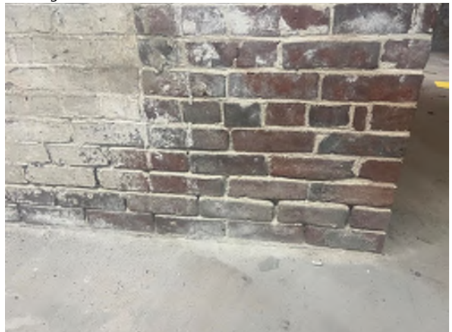
Image 228: View of deteriorated mortar joints at the base of a masonry wall in the basement.
