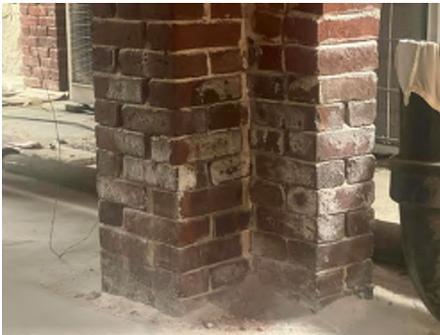
Image 227: View of deteriorated mortar joints at the base of two (2) intersecting masonry piers.
