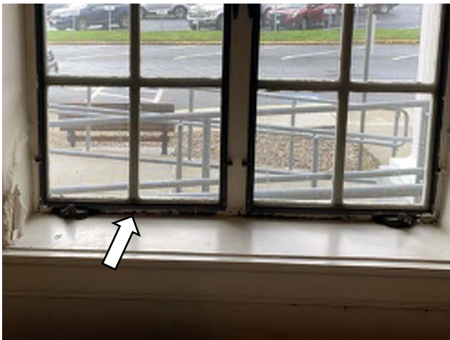
Image 49: Interior view of peeling paint below window.
