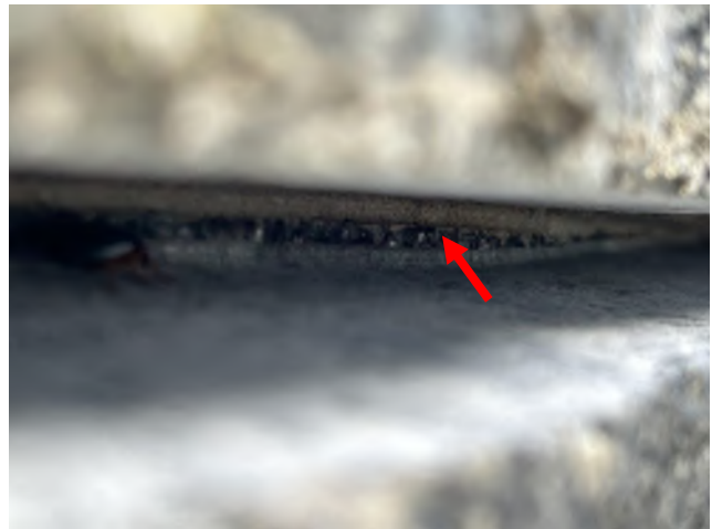
Image 250: Closer view of the previous image shows bedding mortar that appeared intact and metal, which appeared to be the spacer.
