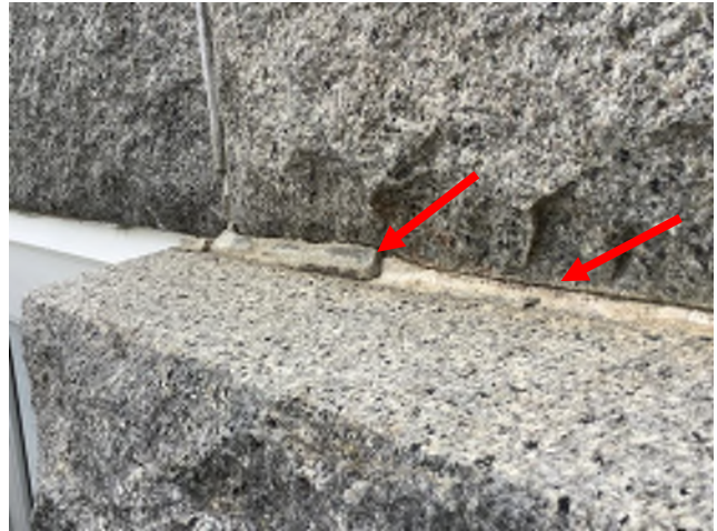
Image 161: Closer view of detached and cracked horizontal mortar between the field of the wall and the foundation.
