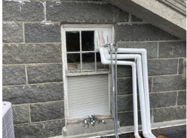
Image 18: View of a window located above the roof line on the South elevation with lower sashed replaced and conduit penetrations.
