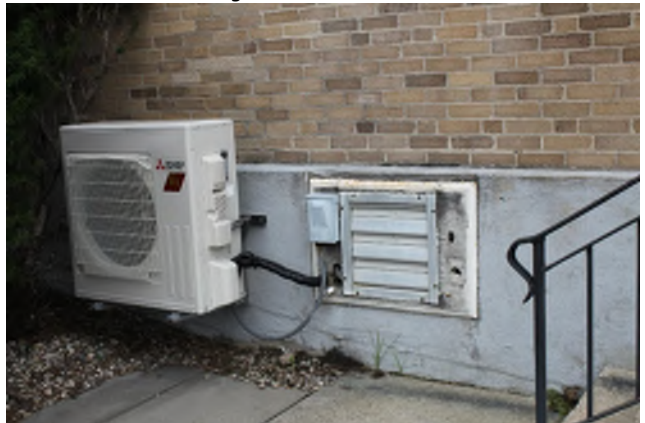
Image 42: Overall view of the infill panel location at South Elevation of one of the 1925 Addition East wing. This location features a number of abandoned and unsealed conduit penetrations.
