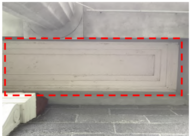
Image 220: Delaminated white paint observed on the soffit above the original building's front entrance.
