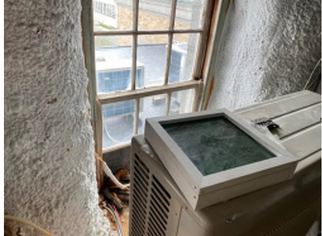
Image 98: Equipment and other items are stored in front of the windows.
