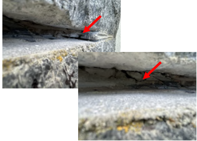
Image 248: Closer views of the previous image show a shallow pointing bead, an apparent separation between the pointing and bedding mortar, and deteriorated (crumbled) mortar in the back of the cut.
