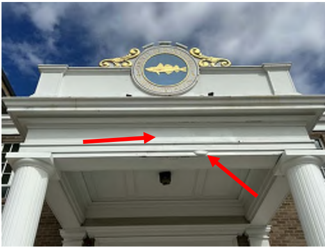
Image 221: View of blistered and faded paint (arrows) on the portico façade at the main entrance of the 1971 addition.
