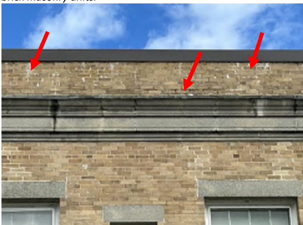
Image 172: Representative view of the parapet shows deteriorated mortar joints and efflorescence.
