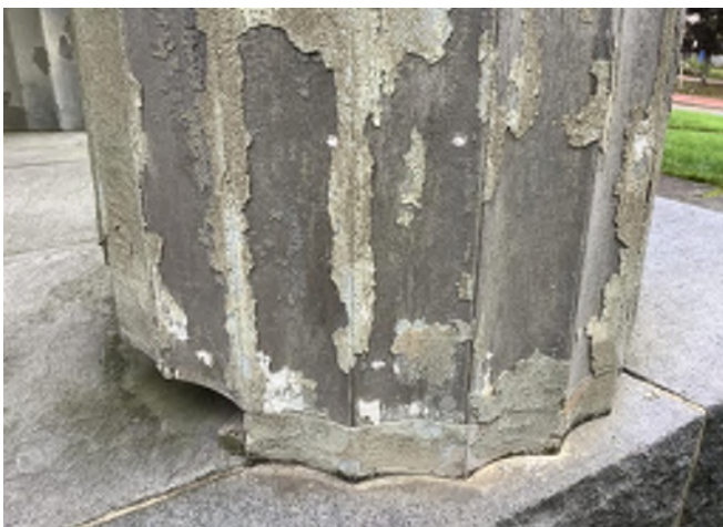
Image 219: Closer view of the previous image shows exposed and missing wood, which was observed at the column bases.
