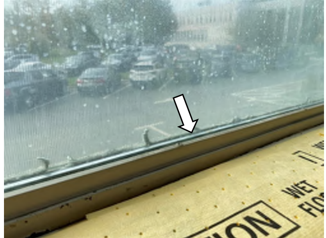
Image 30: The arrow indicates the glazing tape seal that was generally observed to be in poor condition. Also visible is the fogging and staining of IGUs common throughout the 1925 Addition.
