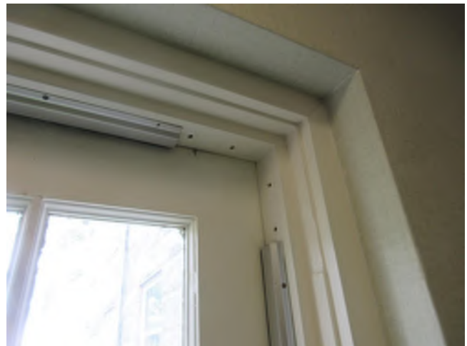
Image 116: Weatherstripping is discontinuous at the head and jamb.
