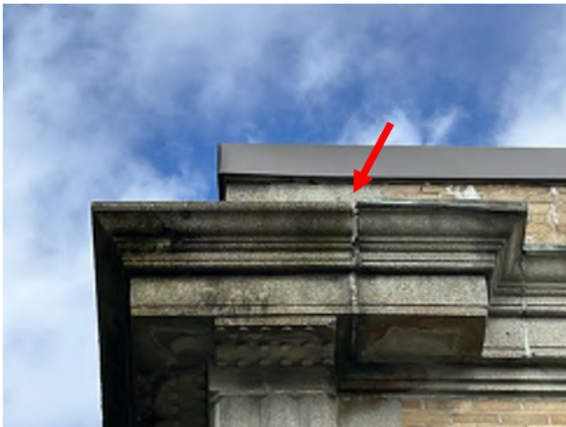
Image 184: Displacement of precast cornice at west end of the south elevation.
