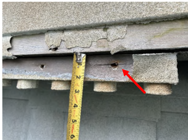
Image 206: View shows a deteriorated (split) decorative wood dentil.
