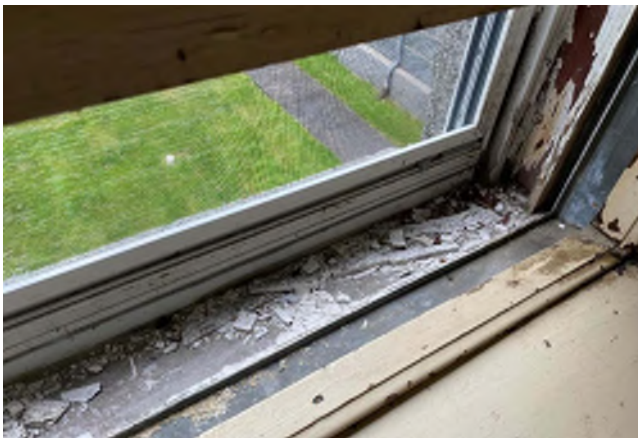
Image 9: Debris from falling glazing putty and paint has typically collected at each window sill.
