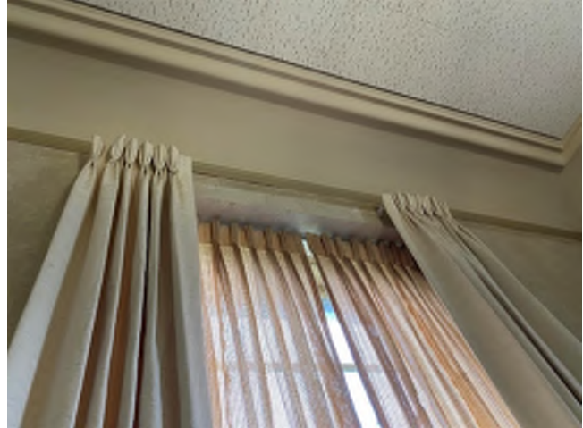
Image 90: Peeling wallpaper was generally noted at the top of the wall around the perimeter of the room.
