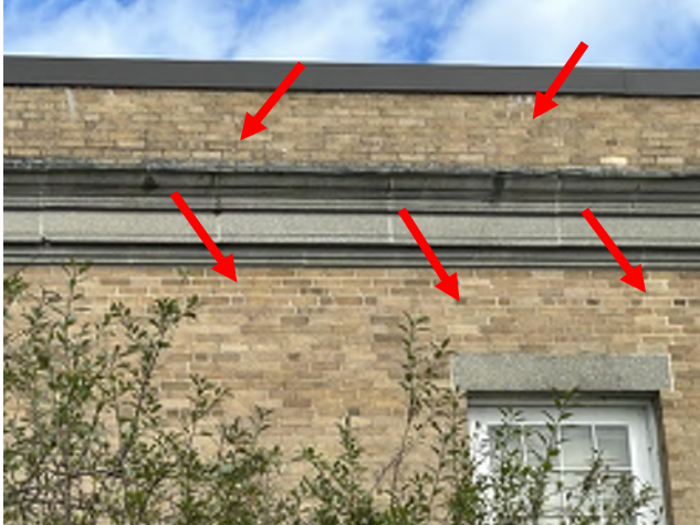
Image 174: Closer view of image above shows deteriorated mortar on the parapet wall, as well as dissimilar colors in the mortar and replacement brick masonry units.
