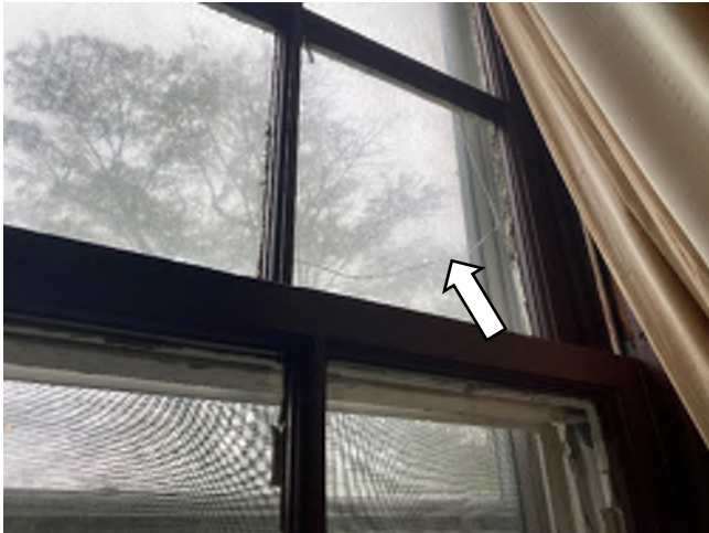
Image 11: The arrow indicates an example of a cracked glass pane.
