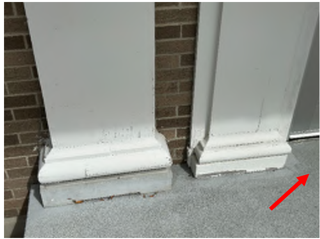
Image 201: Cracked concrete and peeled paint.
