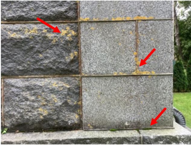
Image 149: View shows vegetative growth on the rock-faced and honed granite elements at the building corner.
