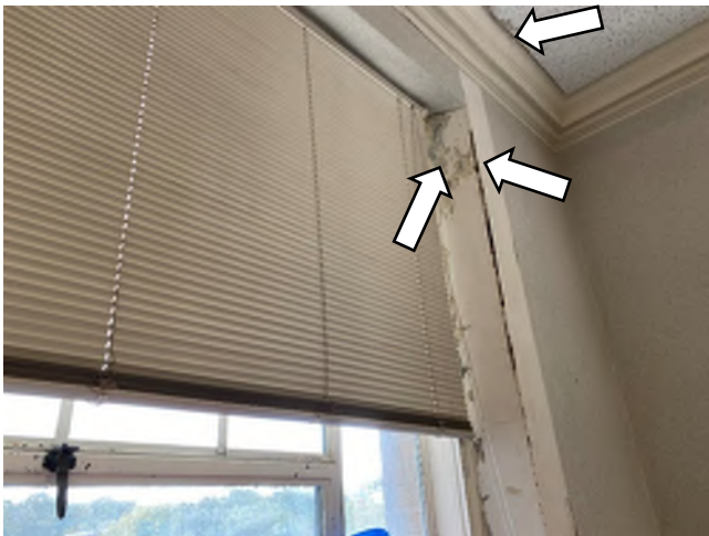
Image 71: One (1) window location exhibited potential previous water infiltration with apparent staining on the ceiling and window jamb, as well as previous wood repairs (arrows).
