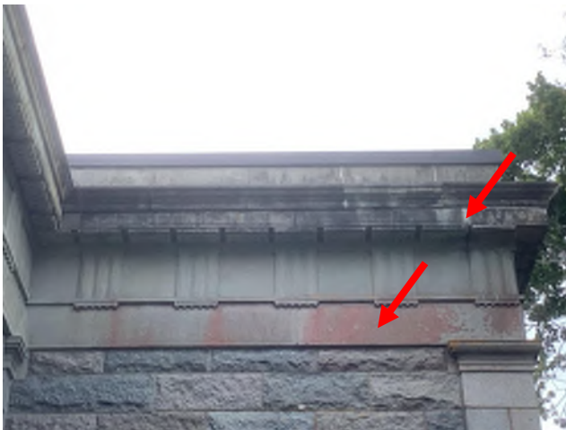
Image 194: Red algae staining and efflorescent staining observed on precast frieze and architrave elements.
