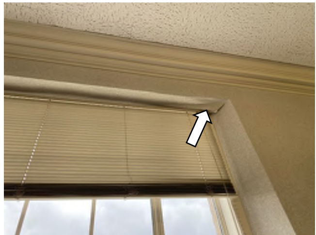
Image 72: An example of peeling wallpaper at a window head.
