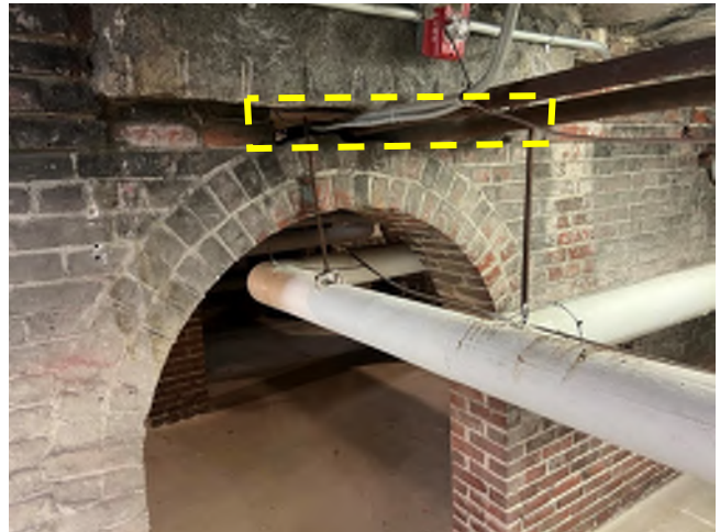
Image 232: View of electrical and plumbing conduits installed above the masonry arch and below the granite block. Note: The dashed box indicates the approximate location of masonry void at electrical conduits.
