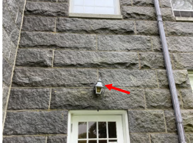
Image 154: Loose lantern observed above an entry door.
