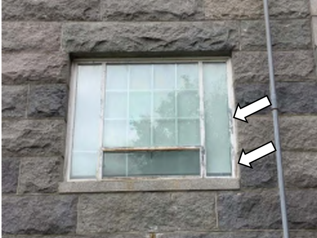
Image 29: Isolated windows exhibited heightened paint defects on the steel frame and wood components (arrows). Rust is also visible on the insect screen at the hopper unit. The hopper unit at this location has one (1) muntin installed, but others appear to be missing or not installed.
