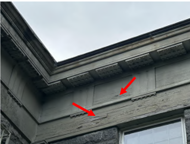
Image 209: View of a displaced wood plank in the architrave and deteriorated wood plank in the frieze portions of the entablature.
