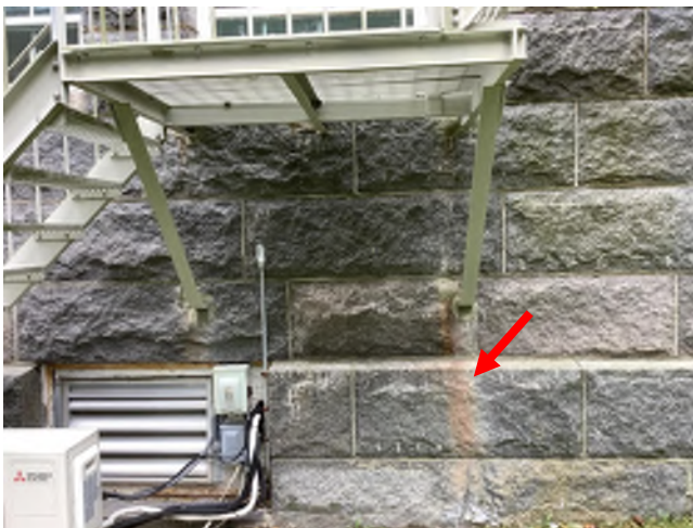
Image 168: Scattered paint and rust staining (arrow) observed below the fire escape on the north elevation of the east wing.
