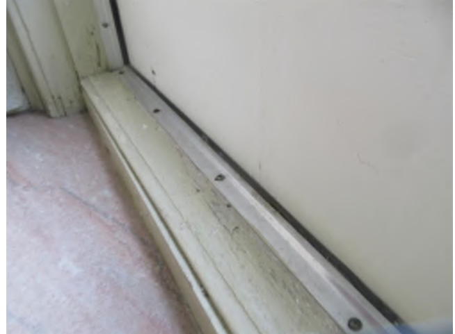
Image 122: Weathered paint was observed on the interior wood surfaces near the threshold level.
