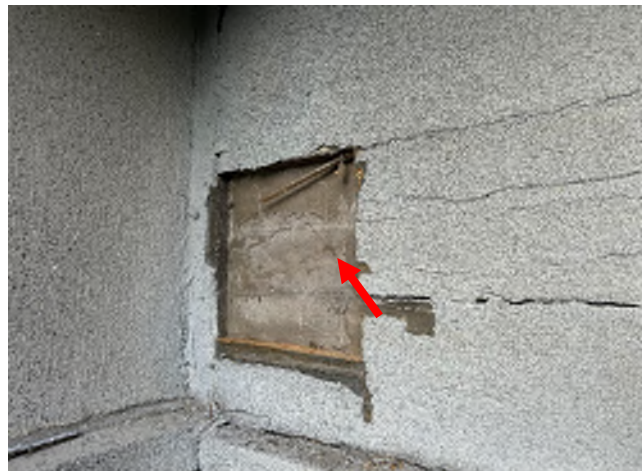
Image 264: Closer view of wood test cut no. 2 shows terra cotta backup directly behind the painted wood fascia.
