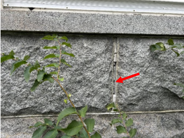
Image 143: Deteriorated/missing mortar joint.
