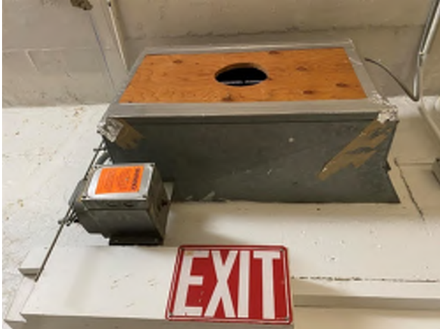
Image 125: The louver above the door appears to be connected to abandoned ductwork.
