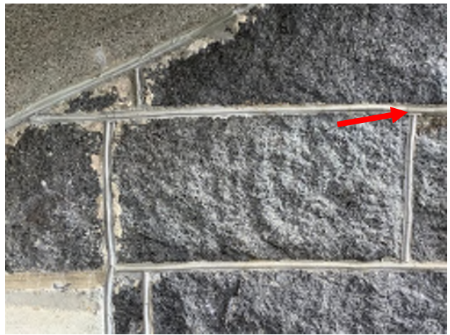
Image 146: South Elevation mortar joint repair and deterioration.
