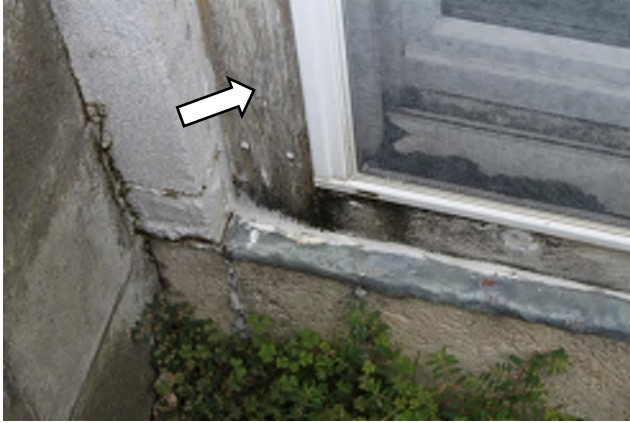
Image 37: The arrow indicates exposed wood blocking at the sliding window units that has lost most of its paint and is showing signs of deterioration.
