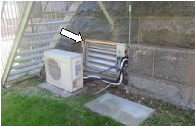
Image 41: Exterior view of the infill panel location on the North Elevation of the East Wing. The arrow indicates a gap that has developed around the displaced infill panel.
