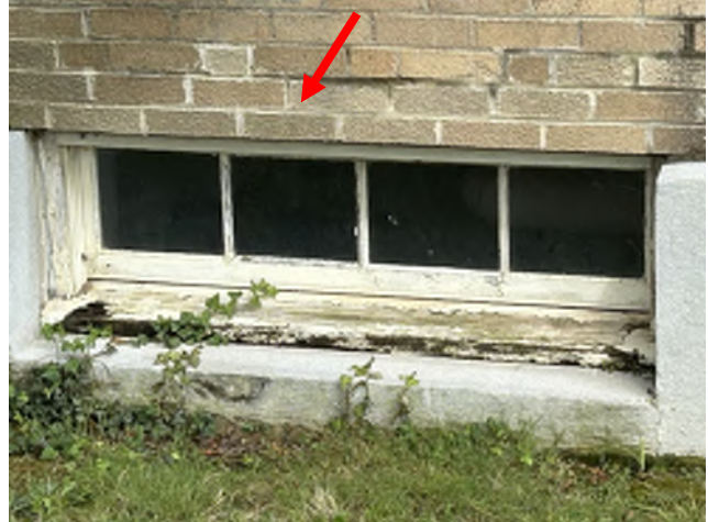
Image 175: Closer view of replacement brick masonry units that have a different color and texture than the majority of the wall.
