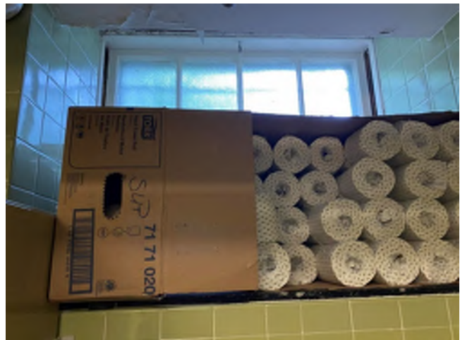
Image 92: View of one (1) of the basement bathroom windows with items stored in front of it.
