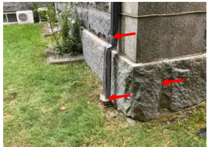
Image 142: View of deteriorated mortar joints in the granite foundation wall (arrow), cracked copper downspout at the elbow (arrow), and grout-filled ground leader (arrow) at the northeast corner of the 1893 addition.
