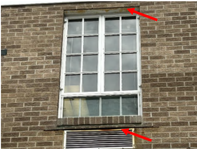
Image 200: Rusted steel lintels observed above a window and louver on the 1971 south elevation.
