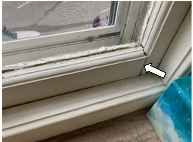
Image 14: The arrow indicates an example of gap opened up between the sash bottom rail and stile.
