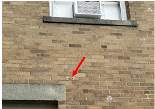
Image 177: Abandoned masonry anchors (arrow) were observed in the masonry wall.
