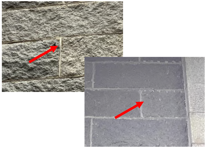
Image 140: Spalling of rock-faced granite.
