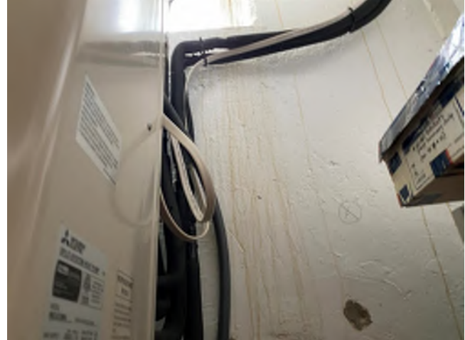
Image 94: Water streaking was evident below isolated window locations in the basement.
