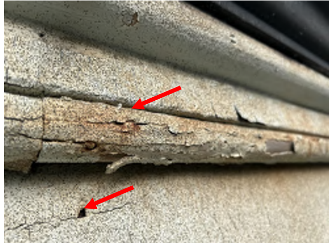
Image 204: Closer, representative view of cracked wood components on the cornice.
