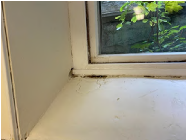
Image 91: Example of damaged plaster at the sloped window sill in basement.
