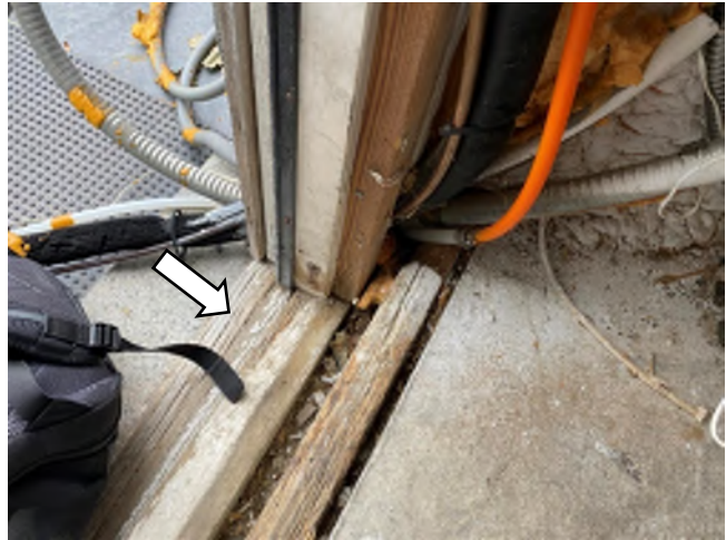
Image 134: Interior view of Door 10 and threshold. The arrow indicates the wood sill that is weatherchecked and deteriorated.
