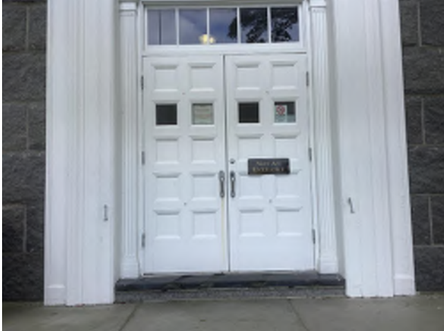
Image 107: Exterior view of Door 3. The arrow indicates a gap observed between the door and frame when the door is in the closed position.
