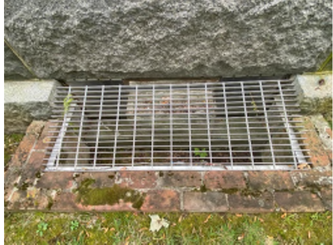
Image 44: At this location on the West Elevation of the West Wing, a metal grating has been installed over the window opening, which has been infilled plywood and what appears to be an abandoned rectangular penetration.
