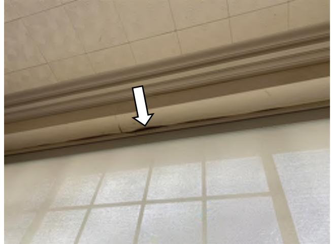
Image 66: The arrow indicates peeling wallpaper observed adjacent to a window head.
