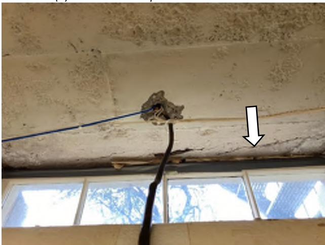
Image 95: The arrow indicates cracking was observed in the concrete floor slab at one (1) of the basement window locations.
