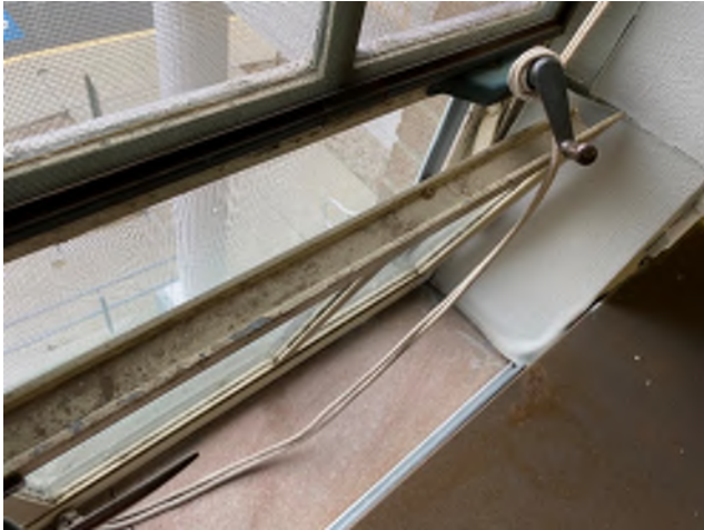
Image 47: Interior view of hopper opening at 1971 steel window. Gale noted a lack of weather stripping.
