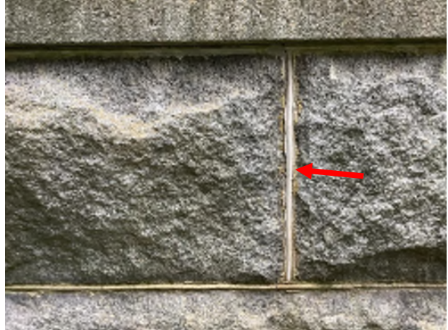
Image 144: Deteriorated/cracked mortar joint.
