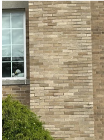
Image 181: Closer view of deteriorated mortar on the chimney.
