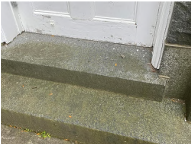
Image 115: Interior view of the Door 2 threshold. No door sweeps or raised threshold are installed. Painted surfaces near the threshold level were observed to be weathered.
