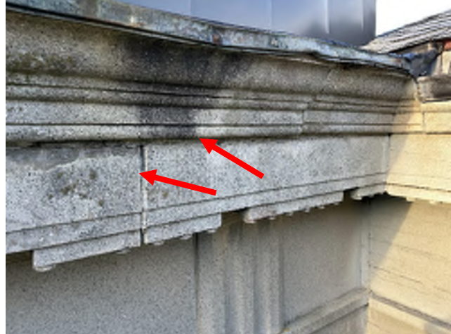
Image 193: Deteriorated mortar observed in cornice elements.
