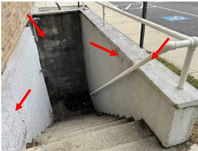
Image 182: View looking down the basement stairs shows delaminated coating on the brick masonry and concrete walls.
