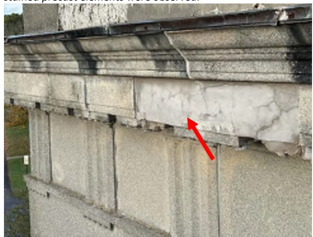
Image 191: Closer view of deteriorated precast repair on the cornice.
