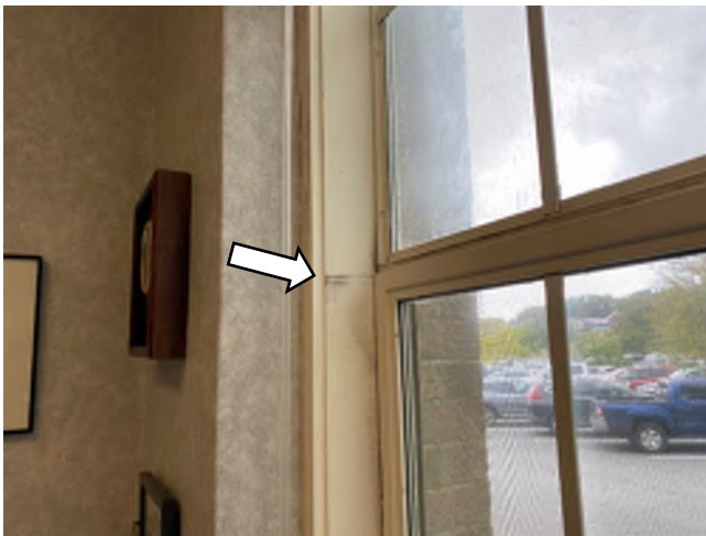
Image 75: An example of paint abrasion due to the hopper window sash rubbing against the jambs.
