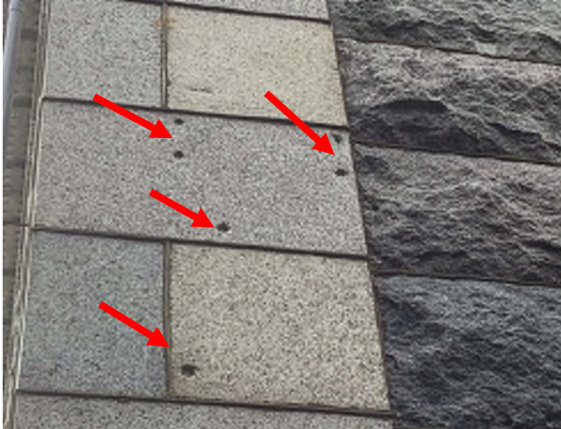
Image 166: Visible holes where embedded anchors were observed in the honed granite at the northeast corner pilaster.
