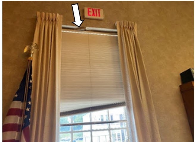
Image 60: The arrow indicates a location of peeling wallpaper.
