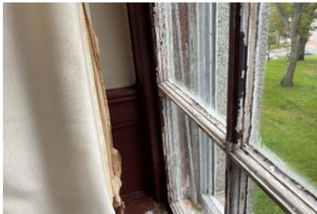
Image 10: Example of interior deteriorated painted wood surfaces.
