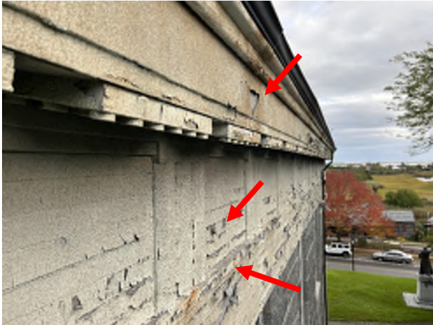
Image 203: Representative view of peeling paint on the cornice, frieze and architrave portions of the entablature.
