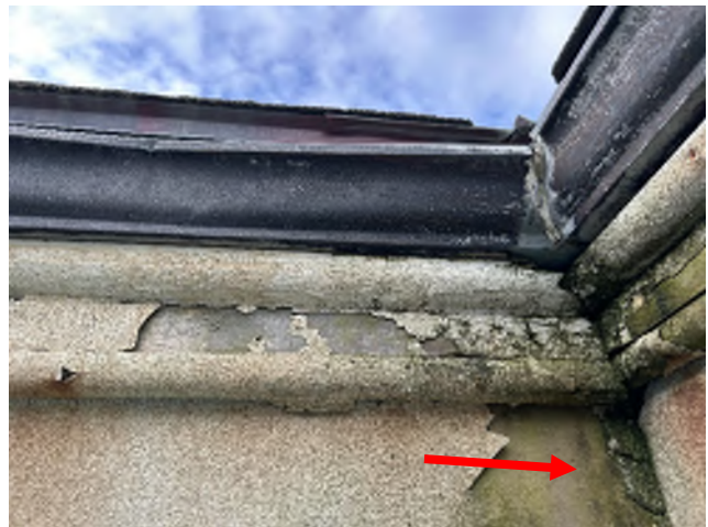
Image 210: View of peeled paint, deteriorated wood fascia board and deformed copper gutter at a cornice.
