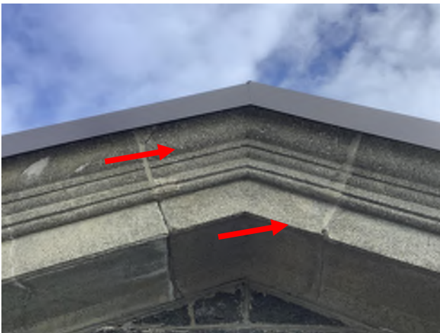
Image 145: Previously repaired, deteriorated and missing mortar on the South Elevation
