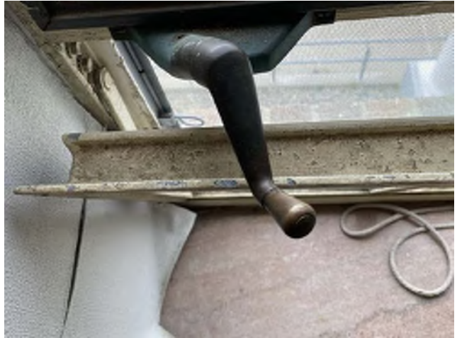
Image 48: Interior view of hopper opening at 1971 steel window. Gale observed peeling paint.
