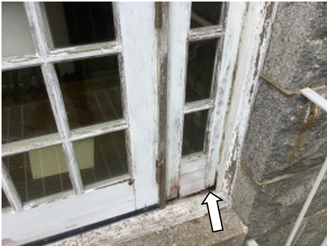
Image 101: Exterior surfaces of the door are experiencing widespread paint deterioration. The arrow indicates visibly warped and decayed wood at the side lite panel.
