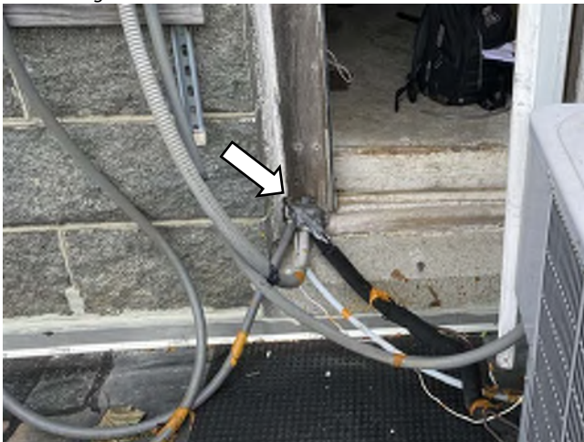
Image 135: The arrow indicates where numerous conduits penetrate through the door frame.
