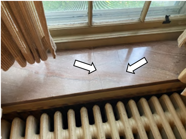
Image 59: The arrows indicate cracks observed in one (1) of the marble stools.
