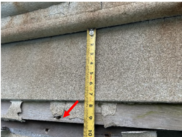
Image 205: Close-up of deteriorated wood trim on the bottom portion of the cornice.
