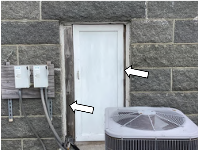
Image 133: Exterior view of Door 10 and associated portico. The arrows indicate exposed wood blocking that is exhibiting severe weathering.
