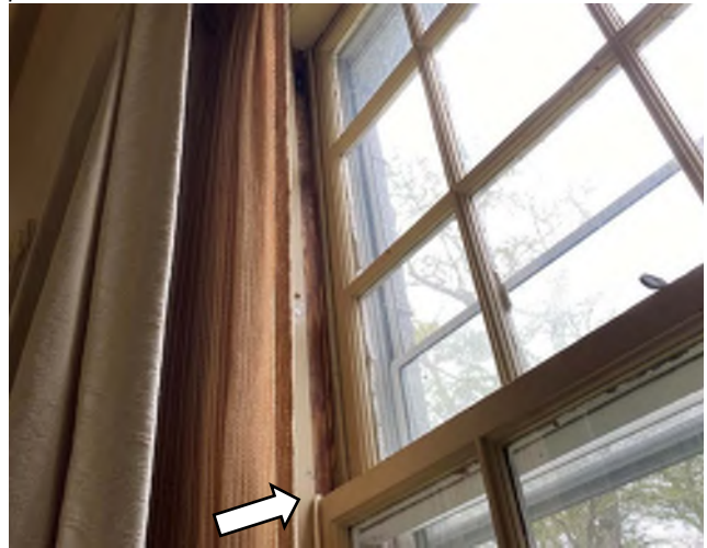
Image 20: View of disconnected upper sash balance.
