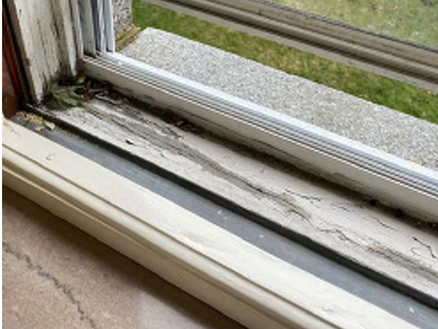
Image 5: Typical peeling paint and weatherchecking at wood sill.
