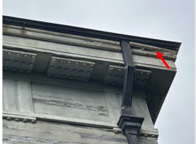
Image 208: Displaced wood trim was observed below the gutter at an isolated cornice location.
