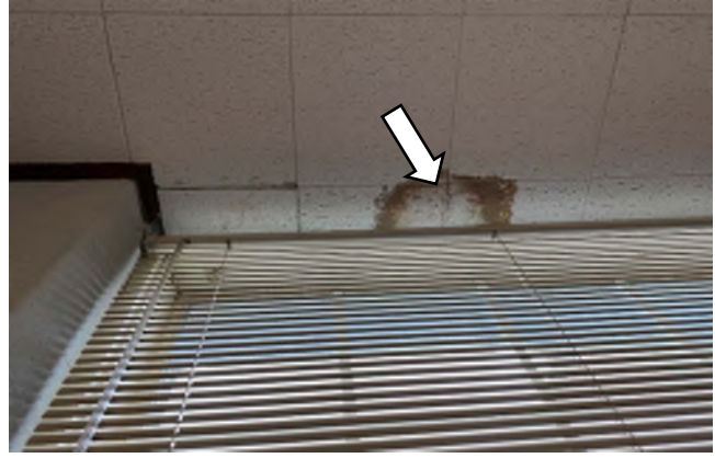
Image 74: Staining was observed on the ceiling at one (1) location in this area. The spline ceiling is installed into the window opening at this location.
