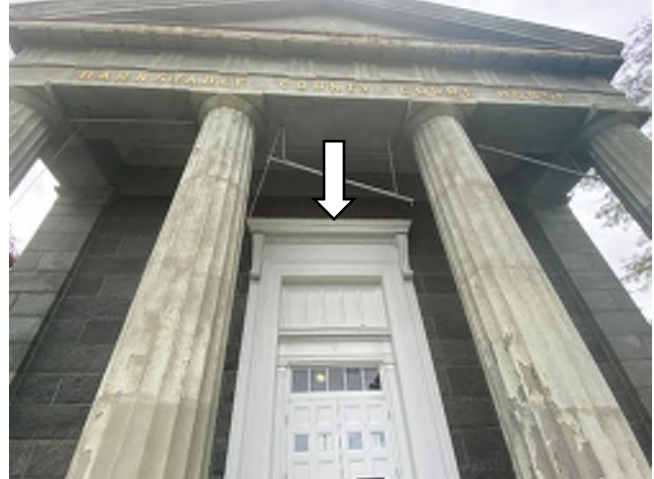
Image 108: Exterior view of ornamentation above the door. The arrow indicates rust staining emanating from the bird screen above the door.
