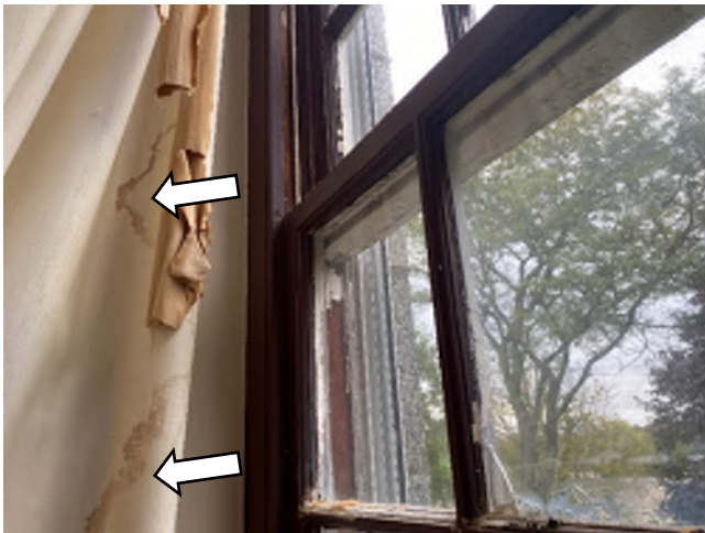
Image 55: The arrow indicates staining on the drapes observed at one (1) window location.
