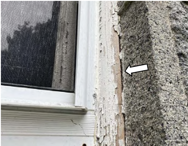
Image 19: Deteriorated cant sealant between wood trim and granite masonry.
