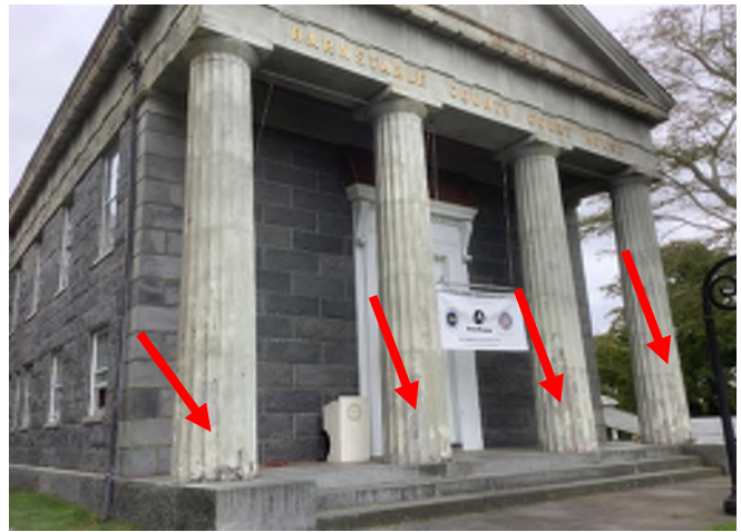
Image 218: View shows deteriorated sand-textured paint on the columns on the original building's front entrance.
