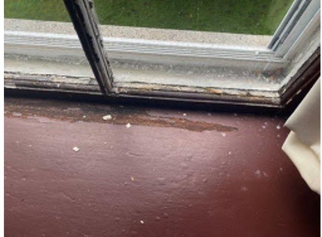
Image 54: Interior painted wood finishes within this space appear to be in worse condition compared to elsewhere on the building.
