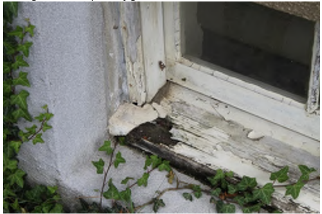
Image 40: The exterior wood components appear to be experiencing heightened deterioration compared to other wood windows on the building.
