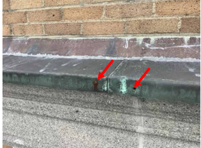
Image 187: Rusted and missing fasteners observed in the copper cornice flashing.
