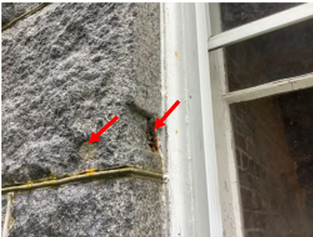
Image 151: Arrows point to a mortar-filled hole (front face) and rust stained granite where an apparent section of embedded iron remains on the jamb return.
