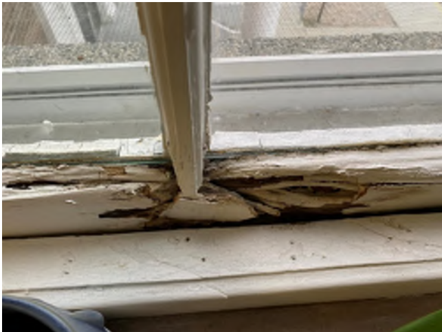
Image 13: A severe example of wood deterioration at a sash bottom rail.
