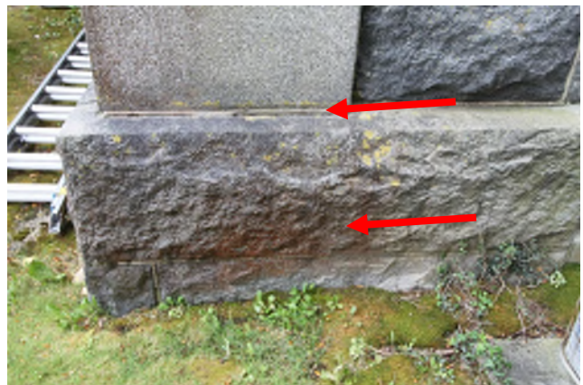
Image 165: Vegetative growth and missing/deteriorated mortar joints.
