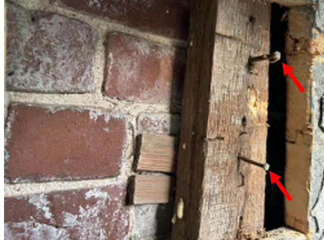
Image 266: Closer view of the previous image shows efflorescence staining and deteriorated mortar in the masonry wall, deteriorated wood furring and rusted fasteners.
