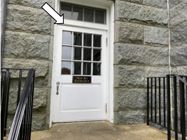
Image 103: Exterior view of Door 2. The arrow indicates a gap observed between the door and frame when the door is in the closed position.
