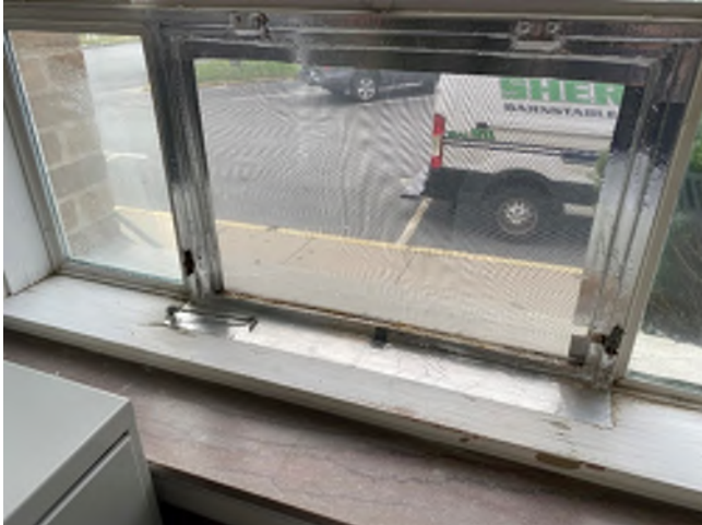
Image 33: At one (1) window location, the hopper unit was taped around its perimeter and the cam handles were missing.
