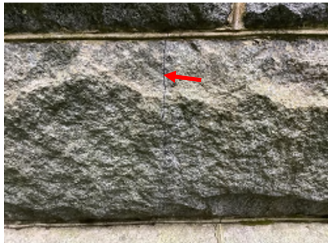
Image 148: Cracked granite element in the field of the wall.
