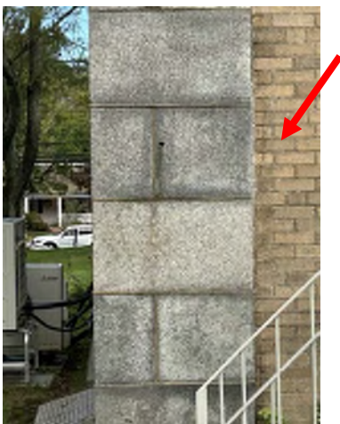
Image 196: Arrow points to abandoned hole in precast pilaster.
