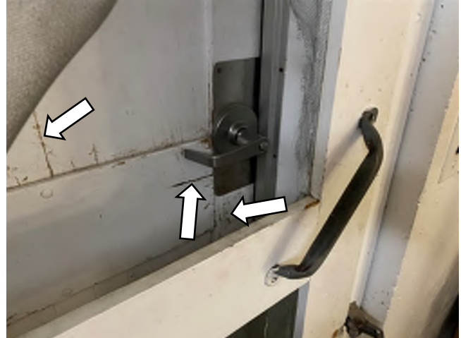
Image 126: The arrows indicate weathering of the interior painted wood surfaces.
