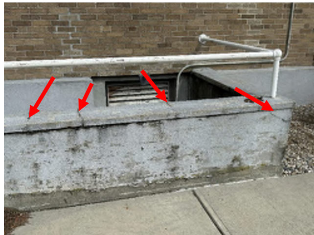
Image 183: Cracks were observed on the concrete wall and coping.
