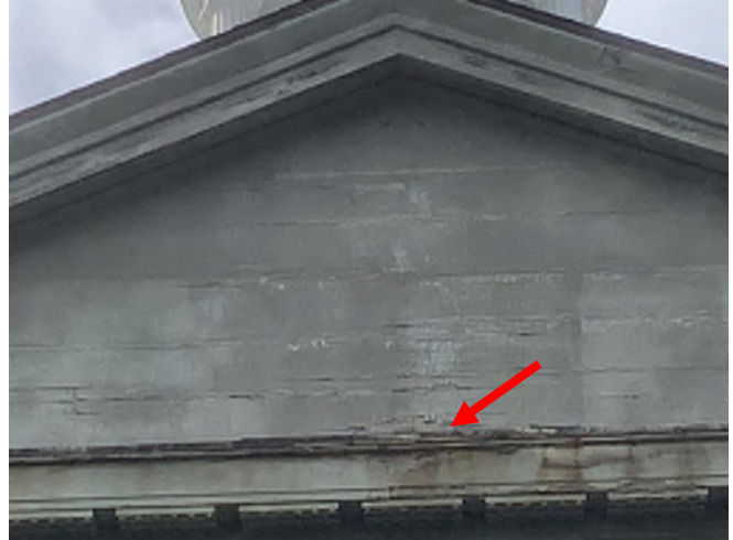
Image 216: Closer view of the previous image shows apparent deteriorated wood elements (arrow).
