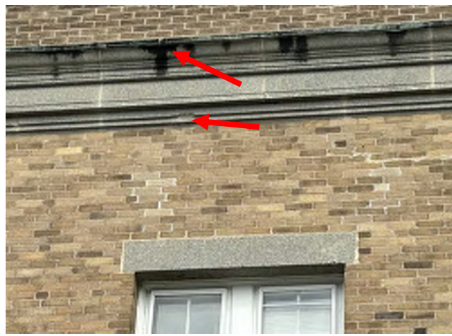
Image 197: Spalled and stained precast cornice elements (arrows) on the south elevation.
