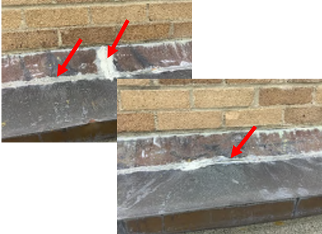
Image 186: Deteriorated solder joints (arrows) observed in the copper cornice flashing.
