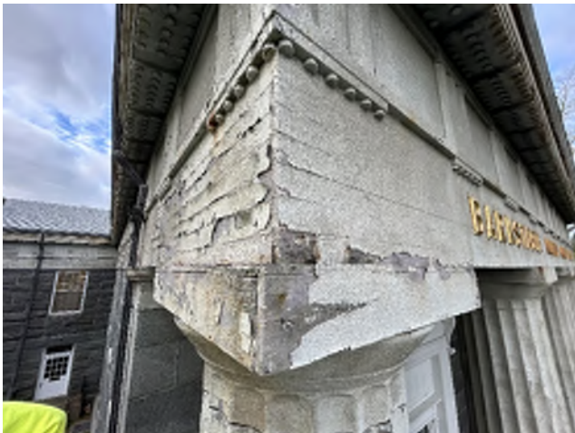
Image 217: Close-up of deteriorated wood trim above a column at the original building's front entrance.
