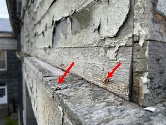
Image 207: Close-up of deteriorated wood frieze components. Note the rusted nails (arrows) that secure the wood.
