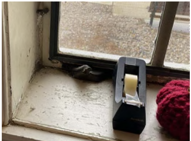
Image 50: View of broken crank at 1971 steel window.
