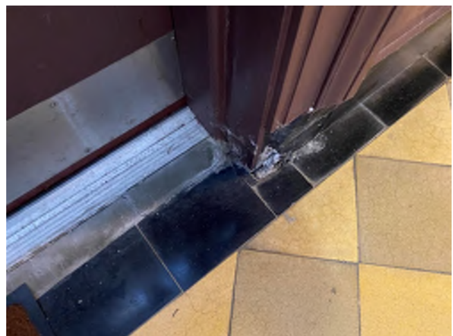
Image 112: The arrow staining emanating from the exterior door hardware.
