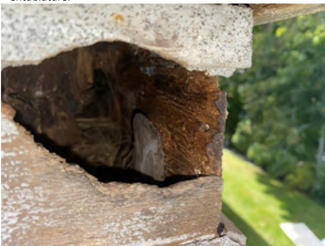
Image 211: Close-up of a missing section of wood trim on top of a pilaster.
