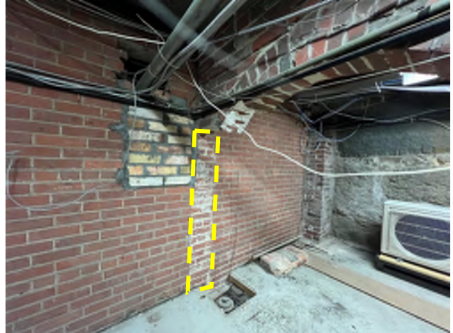
Image 234: Closer view of the missing masonry pier in the southwest corner of the 1831-1832 building that supports the masonry arch. Note: The dashed box indicates the approximate location of masonry pier.
