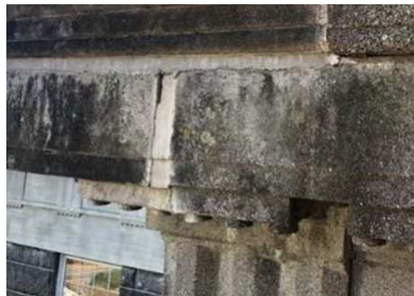
Superior Courthouse – Cornice Stone Failure
