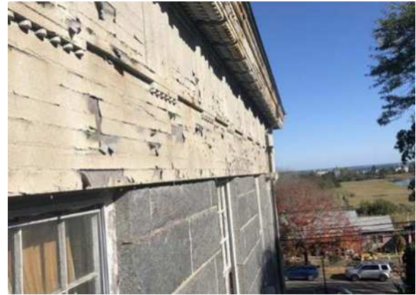
Superior Courthouse – Wood Cornice Paint Failure
