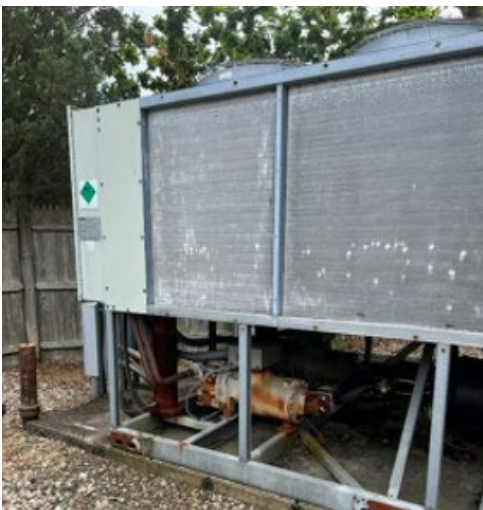
Air-Cooled Chiller Mounted at Ground Level
