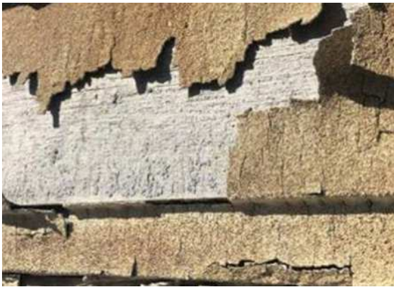
Superior Courthouse – Wood Cornice Paint Failure 2
