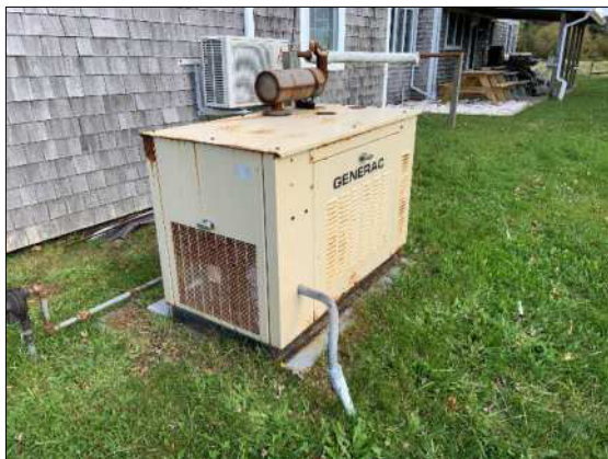
Generator to be replaced
