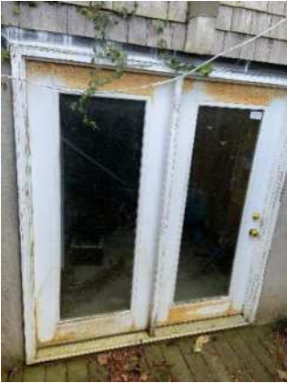
Basement door that floods/rotted decking
