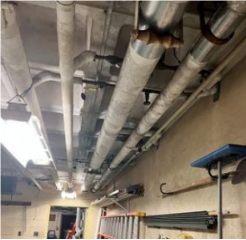
Hot and Chilled Water Distribution Piping in Basement
