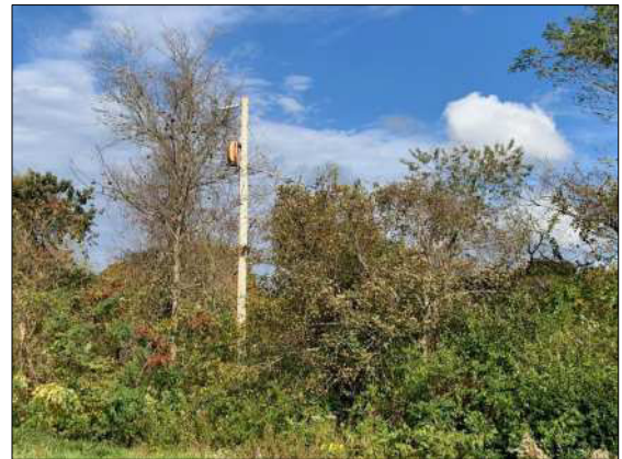
Overgrown utility/electrical services
