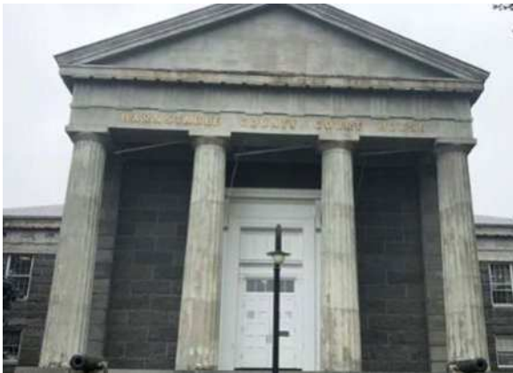
Superior Courthouse – Column Paint Failure
