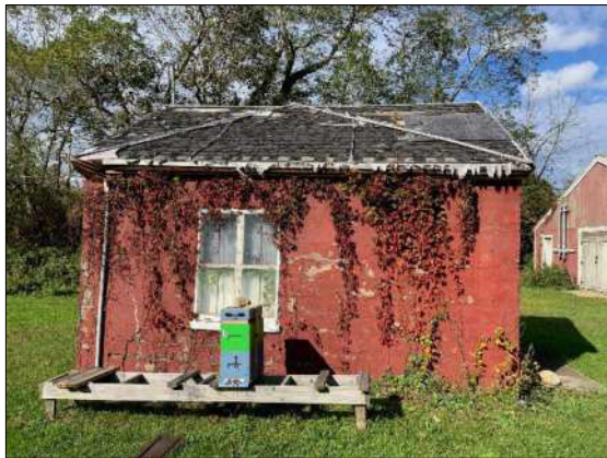
Egg Washing House in need of new roof (this structure houses electrical panel/infrastructure)
