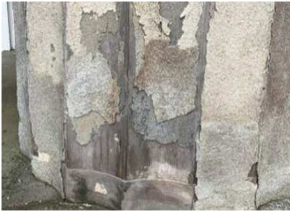
Superior Courthouse – Column Paint Failure 2
