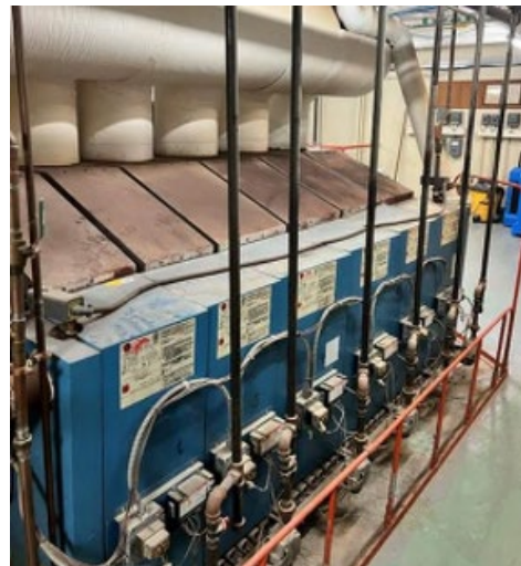
Gas Fired Modular Boilers in Basement
